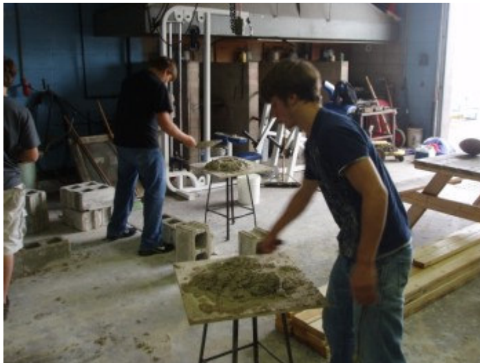
Brett Daniel is working the mortar to get it to the correct consistency. We use lime, sand, and water for our reusable Mix and we need to keep the mortar fairly wet to get the best results.
