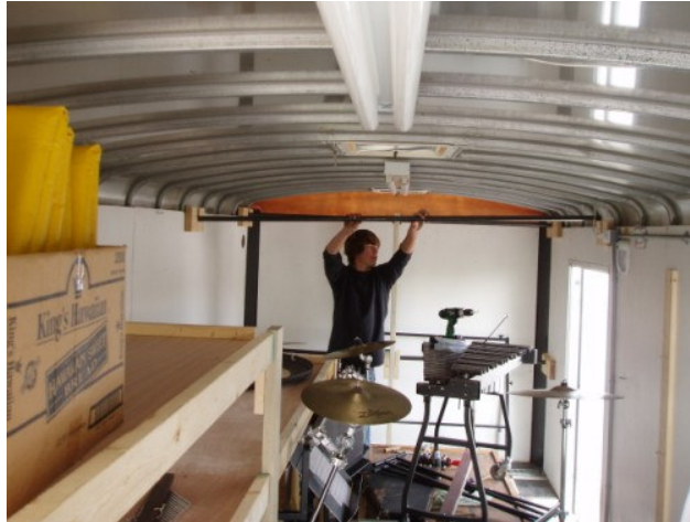
Here is Foster Harrison putting in a second full rod assembly. You can see the door on the right. There is a full rod in front and behind the door. There are two half-rods in front of the door as well.
